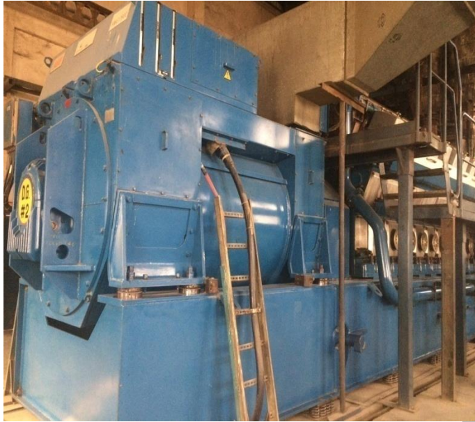
Photographs 2 x 6.2 MW Wartsila
